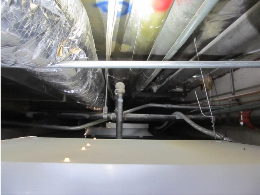
Typical MEP hung from the underside of the slab
