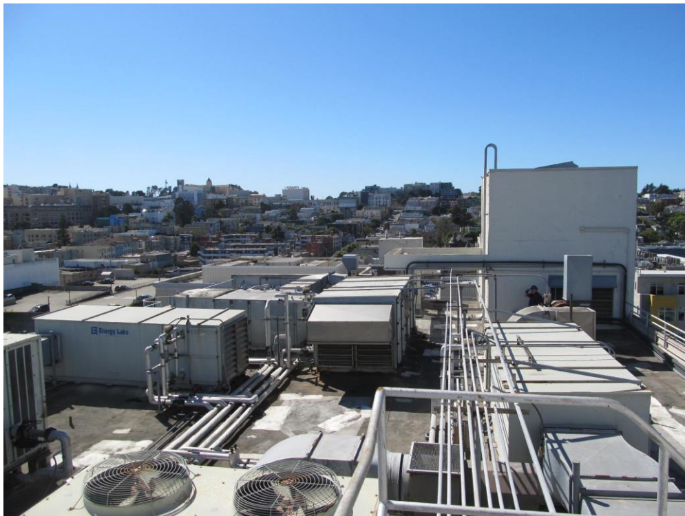
Mechanical equipment at the Main Tower roof (looking west)
