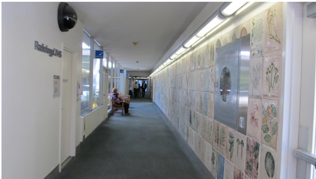
Corridor in the Administration Building leading to the Main Tower. The primary shear wall is on the right (looking north)
