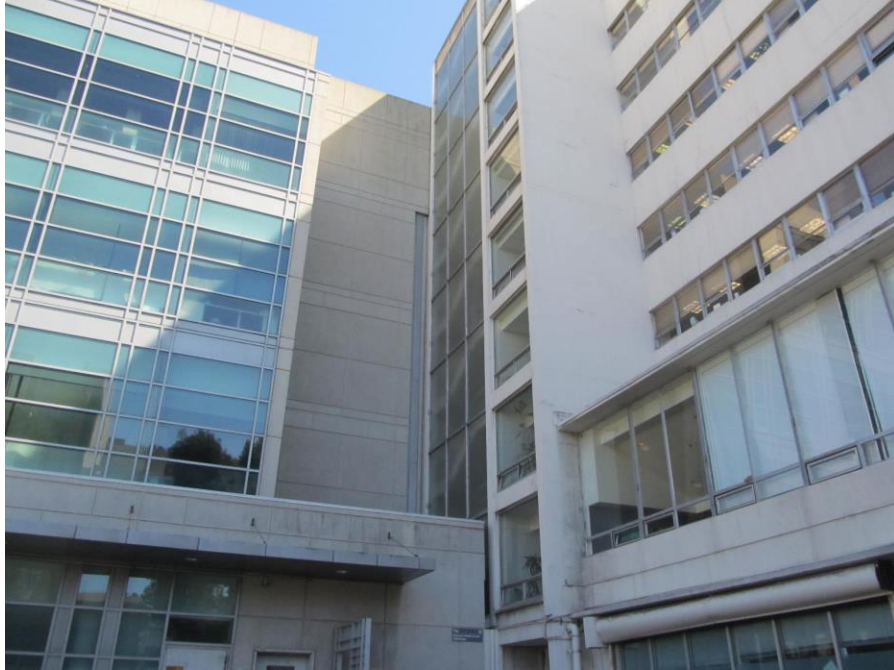
Seismic joint between Building J and the Cancer Research Building (looking southeast)
