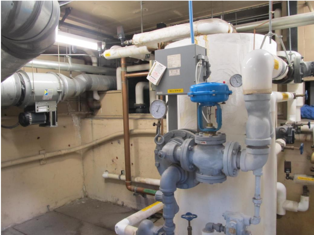
Mechanical room at the first floor (looking northwest)
