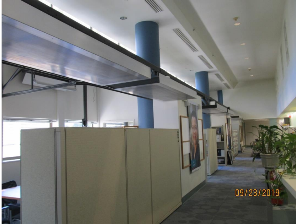
Two-story tall concrete columns at the second floor of the Main Tower (looking southwest)
