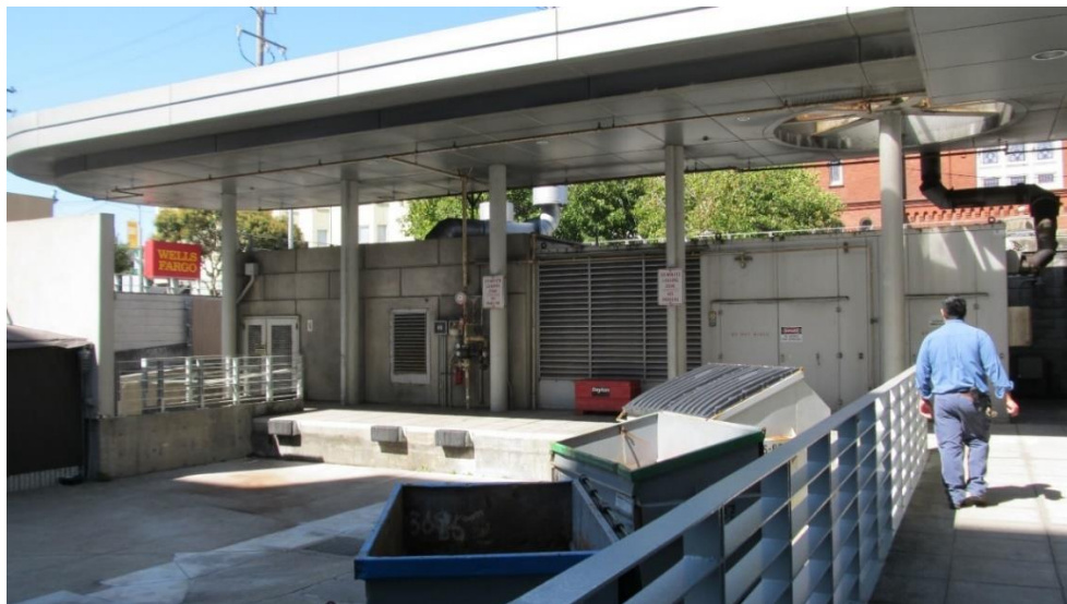
Exterior mechanical room with gas-fueled equipment (looking northwest)
